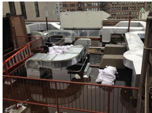
Corridor Roof Top Unit with Heat Recovery
