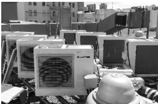
Rooftop air to water heat pumps.
