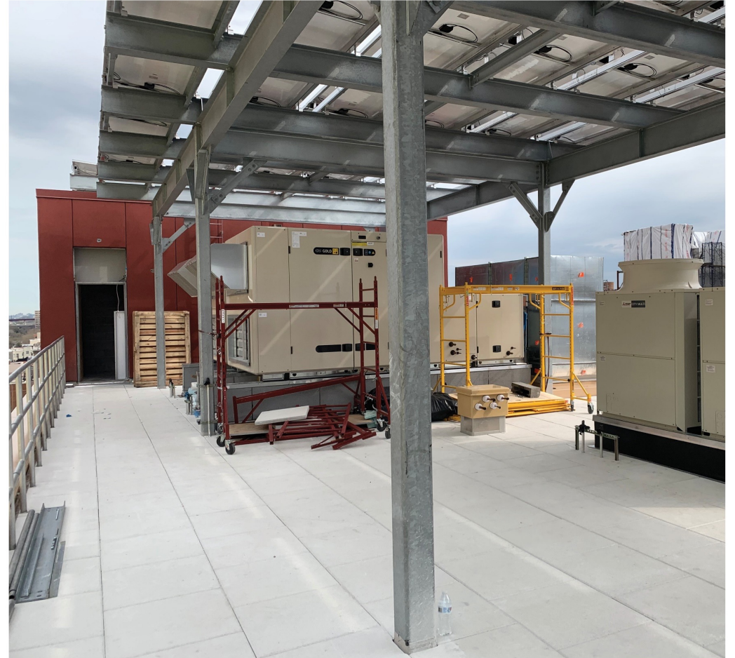
ERVs INSTALLED ON ROOF
