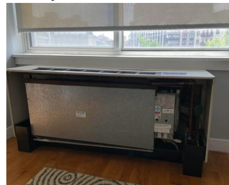
Hydronic Heat PTHPs
